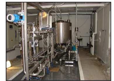
Pictures of various Backflow Prevention Class 4, Class 2 and Class 5 (Air break to tank).
