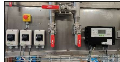
Pictures from various welded water installations from both prefabrication process and from site installation.
