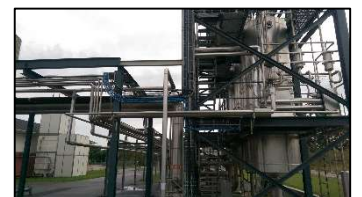
Pictures of tool set for controlling the protective gas, pharma piping, Condensate piping and pipe system for distillation of Ethanol for an API factory.
