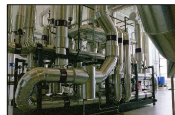
Pictures of different Piping Projects.
