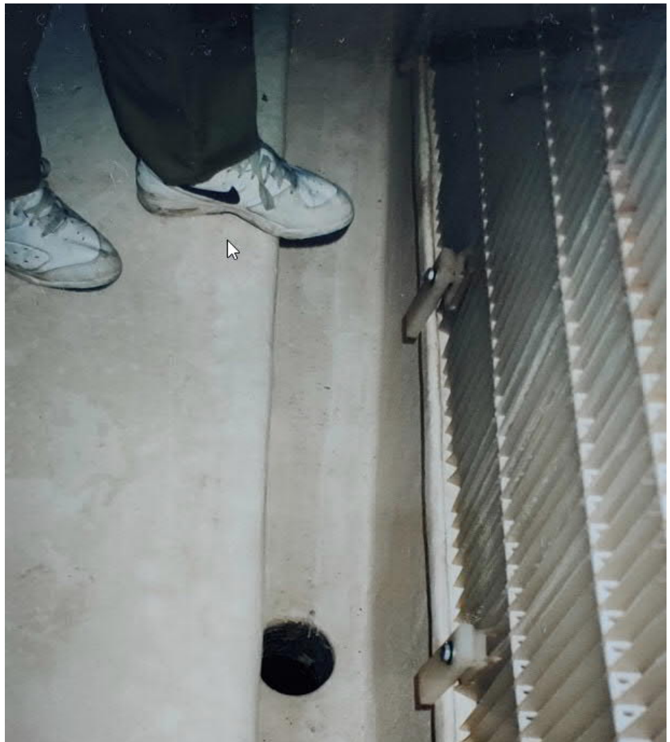
Clean Ducting after De-Mister as the Moisture has been removed.
