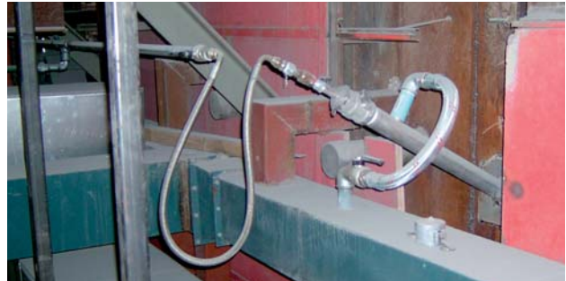
Water injection nozzles mounted through boiler casing and brick wall. Nozzle is cooled with compressed air.
