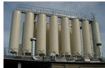
Pictures from Ethanol Distillation and Reception Station, Spray Drying Chamber with Explosion Damper & Duct and Storage Facility for Special Oils.
