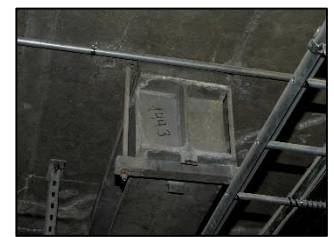
Pictures from ARC (Amagerforbrædningen) where platforms were designed and delivered as EPC.
