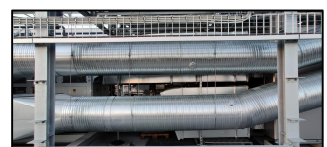
Pictures from installation of both steel structure, General Installations and Solar Panels on roof top.
