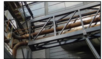
Picture A) Structure for Cyclone B) Pipe and Platform Support C) Distillation Tower and Pipe Bridge and D) Pipe Bridge at Waste Incineration plant – Vestforbrændingen www.vestfor.dk
