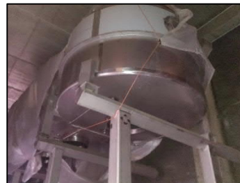
Pictures from a Lactose factory with arrangement and installation of fluid bed during construction.
