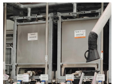
Top: Picture of doubled Walled Plastic Tanks for API Below Standard Stainless Steel IBC Containers were used for storage.
