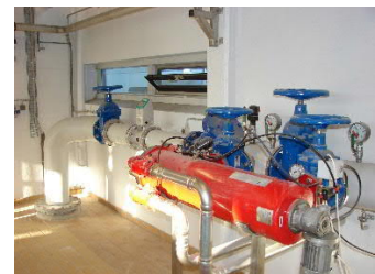
Pictures from Installations on top of Water Ressoar..
