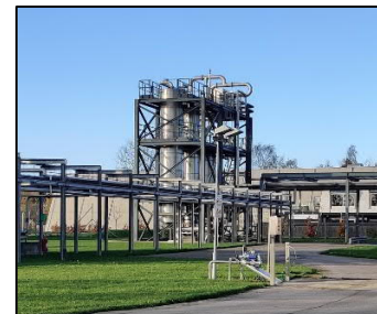
Pictures from Ethanol Storage & Distillation in relation to API-factory (DK) for Dextran production.
