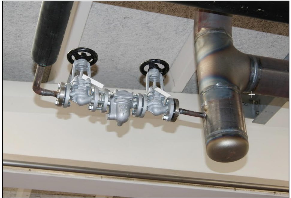
Example of a Steam Drain with Thermostatic Steam Trap. From Steam distribution on an API – Active Pharmaceutical Ingredient – factory in Denmark.
