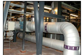
Pictures from Large Scale Heat Pump Installation at Vestforbrændingen (DK) – www.vestfor.dk with Salt Based Heat Pumps. P-Engineering also handles Ammonium Heat Pump Installations.
