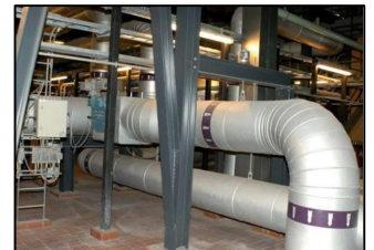
Pictures from Large Scale Heat Pump Installation at Vestforbrændingen (DK) – www.vestfor.dk with Salt Based Heat Pumps. P-Engineering also handles Ammonium Heat Pump Installations.
