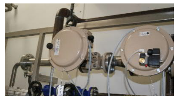
Pictures from CIP Unit at API factory. Pharma Grade Tube & Shell Heaters with Steam were used for Loop Heating.
