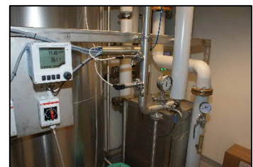
Top: Add-on Unit to existing facility. Middle: New WFI-Unit. Middle: Loop Outtake in Lab @ AGC Biologic. Bottom: HPW unit for Gentofte Hospital.
