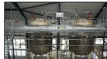
Pictures from a Fermentation Installation with room for 9 Fermenters and 2 off installed when picture was taken. Picture from an API-factory producing Dextran.
