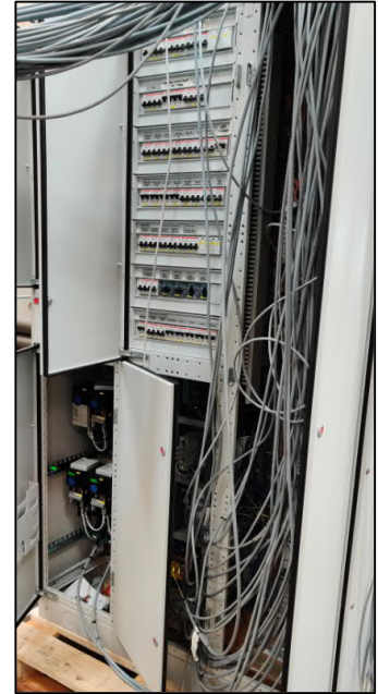
Example of a MCC Panel under Cabling installation during a FAT-test of a unit.
