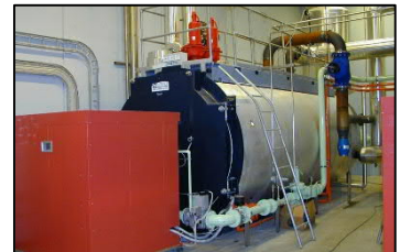
Pictures of a Burner Supply Stations for Large Utility Boiler Burner and a smaller Industrial Boiler Station at a dairy.
