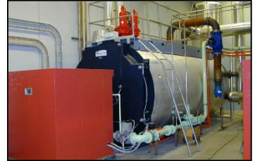
Pictures of a Burner Supply Stations for Large Utility Boiler Burner and a smaller Industrial Boiler Station at a diary.
