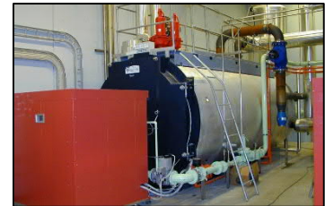
Pictures of a Main Gas Line for Industrial Steam Boiler Plant and a Gas Ramp for at Hot Water Boiler.
