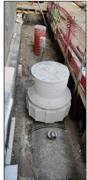
Pictures of Pharma Grade Waste Piping and an overview of vessel in the ground with buoyancy protection straps.
