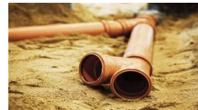
Pictures of various Sewage installation in the ground.
