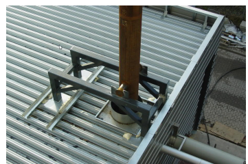
Pictures of Heat Exchanger Unit and from exceptionally large Cooling Installation with 2MW Heat Exchangers
