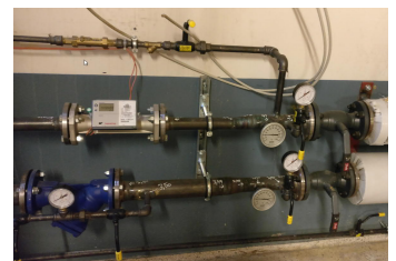
Pictures from the pre-fabrication of a DN100 District Heating Mains Installation and an onsite fabricated DN40 District Heating Mains Installation.
