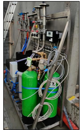
Pictures of Unit with Guldager Equipment for De-Scalled 6°dH and 0°dH as well as Osmosis Unit. Unit lifted in during early Erection Phase.
